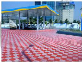
BPCL PUMP PROJECTS
